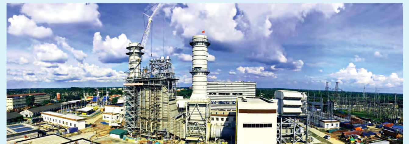
古拉绍燃机电站项目全景图 Panorama of the 365MW Combined-cycle Gas-turbine Power Station Project in Ghorasal, Bangladesh
