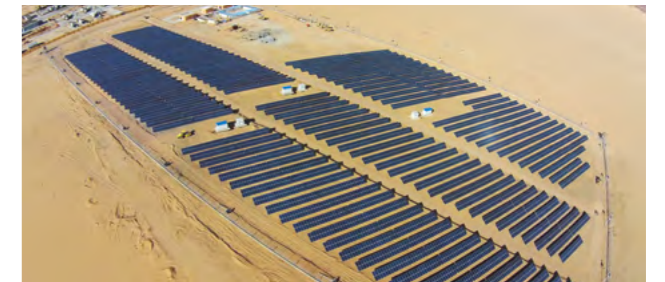
阿尔及利亚 25MW 光伏电站项目全景 The panorama of the 25MW Photovoltaic Power Station project, Algeria
